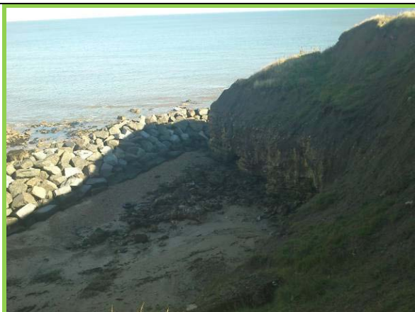
Continued slumping of upper cliff behind rock armour berm. (Asset Ref. No. 121AC901C0103C01)
