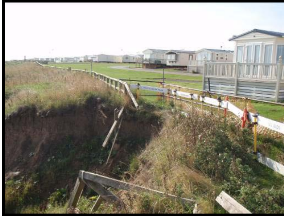
Cliff failure near north end of caravan park. Photo from 2010 report. (Asset Ref. No. 121AC901C0301C01)
