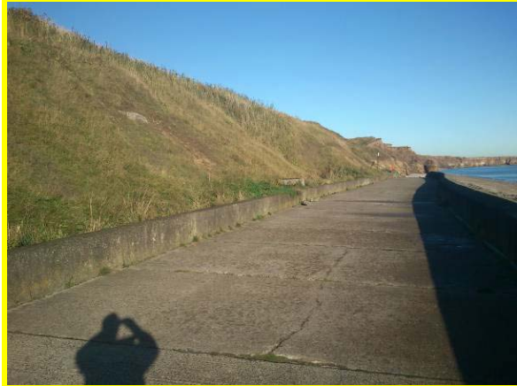
Cracks to promenade with vegetation growth. Well vegetated cliff to rear. (Asset ref. No. 121AC901C0102C01)
