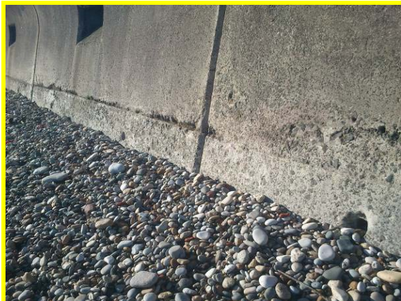
Minor abrasion damage to lower wall (Asset ref. No. 121AC901C0102C01)
