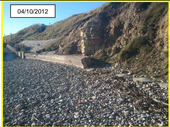
Minor outflanking at interface with wall. (Asset ref. No. 121AB901B0804C01)
