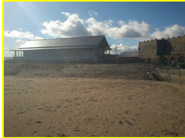
Dressed masonry revetment slope with new marina building to rear. (Asset Ref. No. 121AC901C0104C05)
