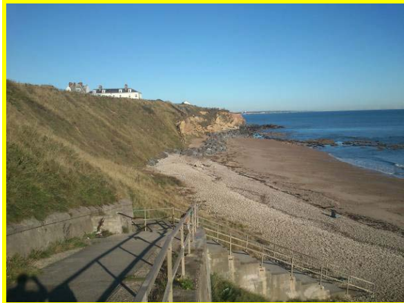
Signs of previous slumping in cliff to north of beach access ramp. (Asset Ref. No. 121AC901C0103C06)
