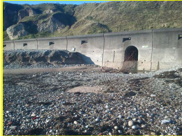
Scour channel at outfall from Seaham Dene (Asset ref. No. 121AC901C0102C01)
