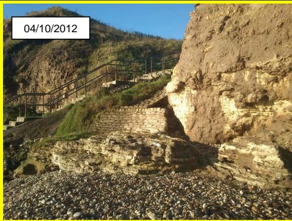
Outflanking at north of steps unchanged from 2010. (Asset ref. No. 121AB901B0804C01)
