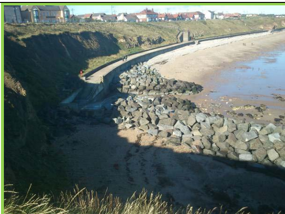
Rock armour protecting headland south of seawall in good condition (Asset Ref. No.121AC901C0103C01)
