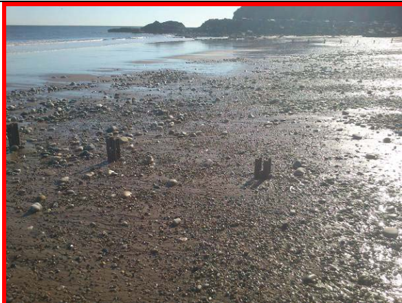
Groyne piles on beach at south end. Recommended to confirm redundant and remove to reduce H&S risks. (Asset ref. No. 121AC901C0102C01)
